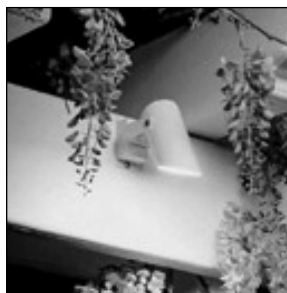
Directional wall-mounted security light in matching wall color
