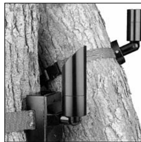
Directional moonlighting and high branching uplighting is achieved using slender fixtures strapped to a tree trunk above eye level
